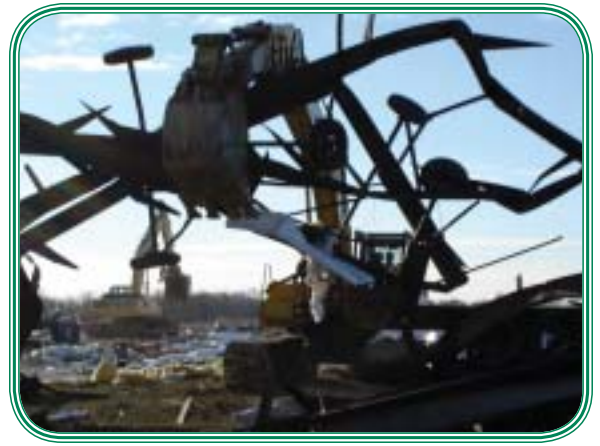
A backhoe picks up a mobile home frame at Eastbrooke mobile home park.
