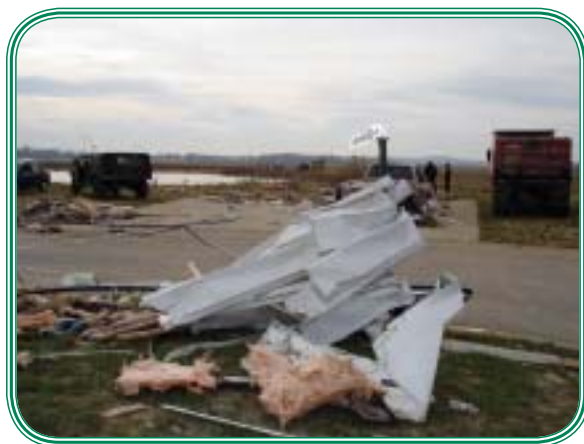
Siding wrapped around the street sign shows the force of the wind (est. 200 mph)
